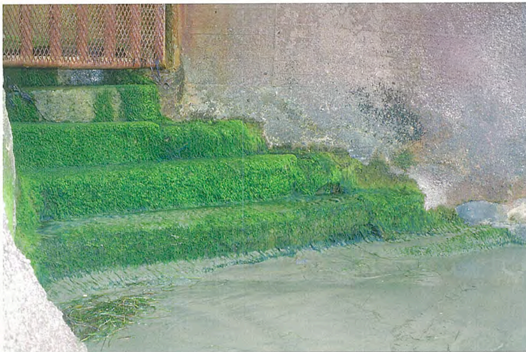
FIG. V-6. SAN DIEGO CO., LA JOLLA. Although seawalls, breakwaters, and other artificial revetments provide habitat, they also impact the coastline (shown here is Ulva lactuca blanketing a concrete walkway down a seawall in La Jolla). Loss of natural shoreline features and habitats, and alteration of the beach-building and excavating functions of the longshore current are significant impacts.
